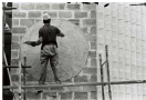
1932: Workers at the site of the new State College in the grounds of the College in the early 1930s.
