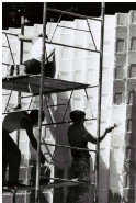
WORKERS ON A BUILDING SITE IN A CITY IN THE SOUTH OF FRANCE (1988)
